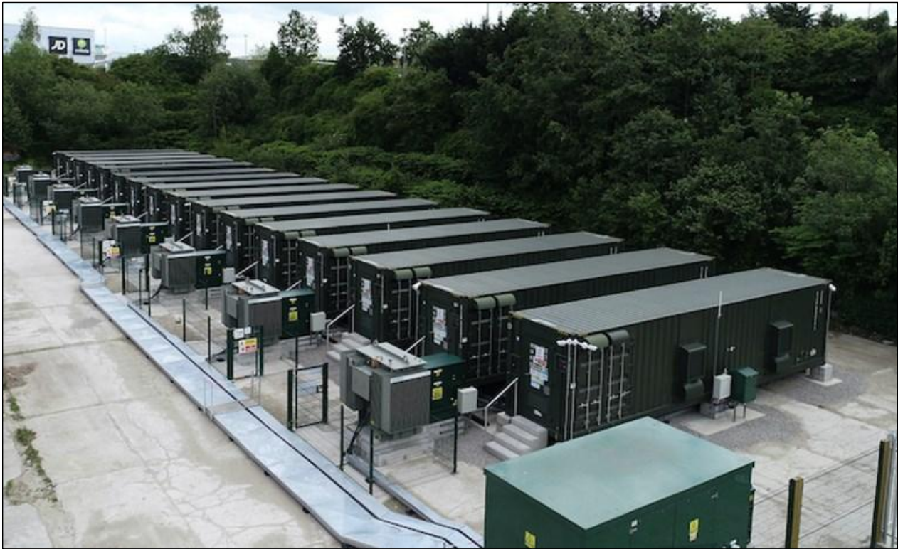
FIGURE 9 Example Anesco battery storage facility (Source: Anesco; https://anESCO.com/blog/2020/10/30/gore-street-energy-storage-acquires-battery-portfolio )
