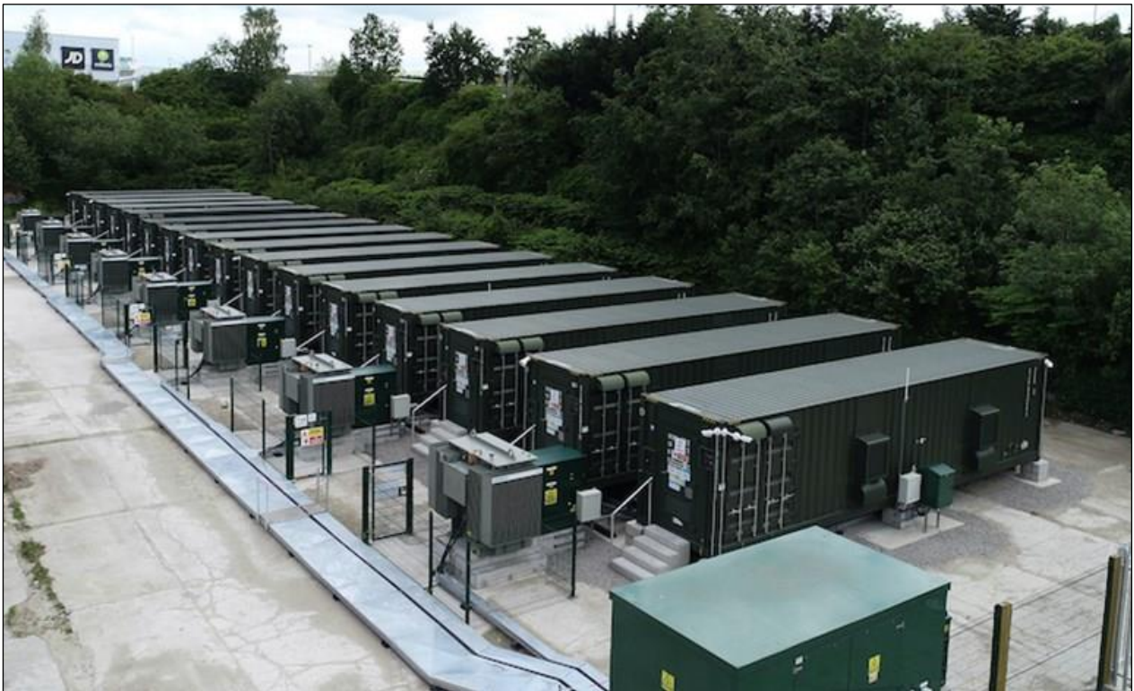
Figure 8. Example Anesco battery storage facility (Source: Anesco, anesco.com/blog/2020/10/30/gore-street-energy-storage-acquires-battery-portfolio/ )
