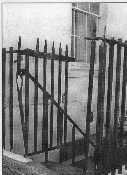
Fortfield Terrace; corroded ironwork in need of restoration.
