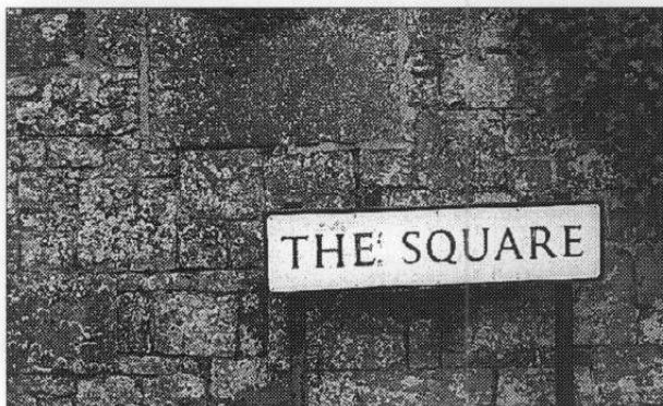
Retaining wall enclosing churchyard. Attractive squared-off, possibly sawn stone in a variety of dimensions, probably mid 19th century; a demonstration of once widespread skills of stonemasonry.
