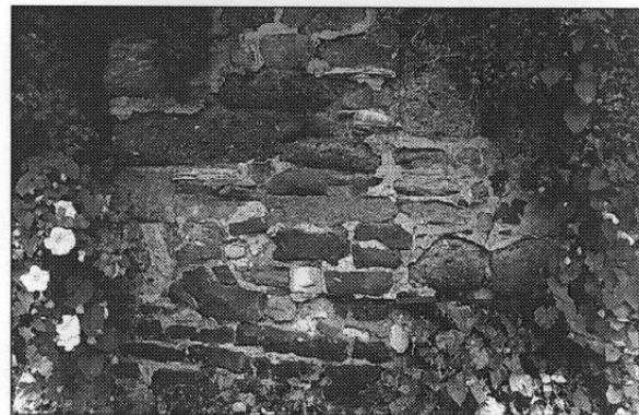
Stone walls, mainly of sandstone conglomerates from local quarries (e.g. Heavitree) are found in several locations. Condition is varied but some sections are in definite need of low key maintenance/repair using the right kind of replacement stone and minimal amounts of soft mortar, preferably using lime.
