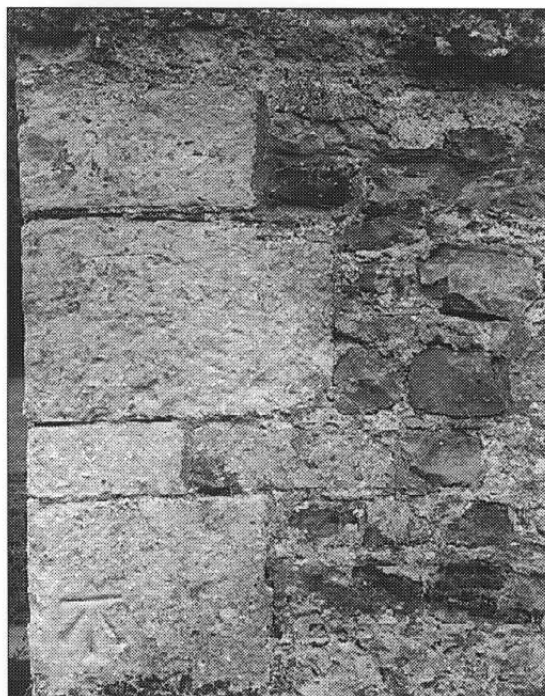
Wall detail of the Parish Church tower showing dressed Beer stone and coursed chert
