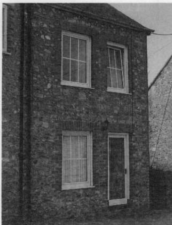
Inappropriate PVCu windows fitted into a key building.
