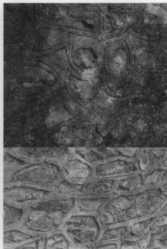
Two examples of re-pointing where cement has been used and obscured the individual stones.
