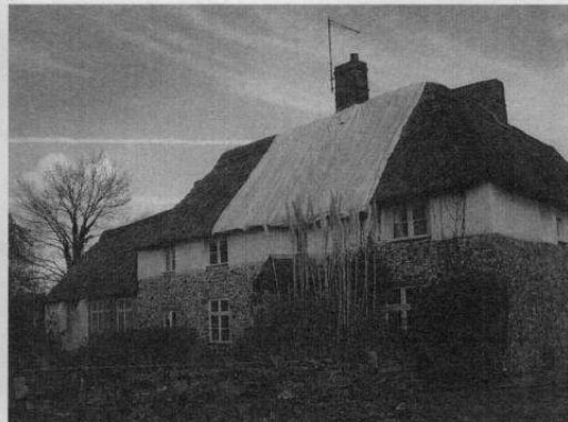
Poor condition of thatched cottages awaiting re-thatching.
