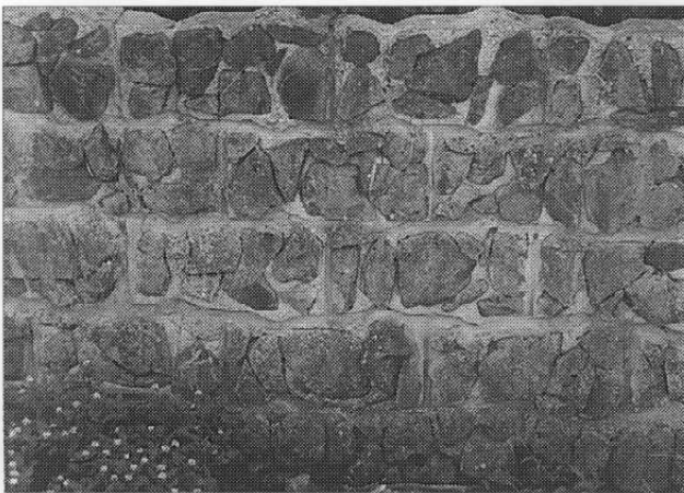
Close-up view of the pre-fabricated stone impregnated concrete wall enclosing the stream along much of its course through the village
