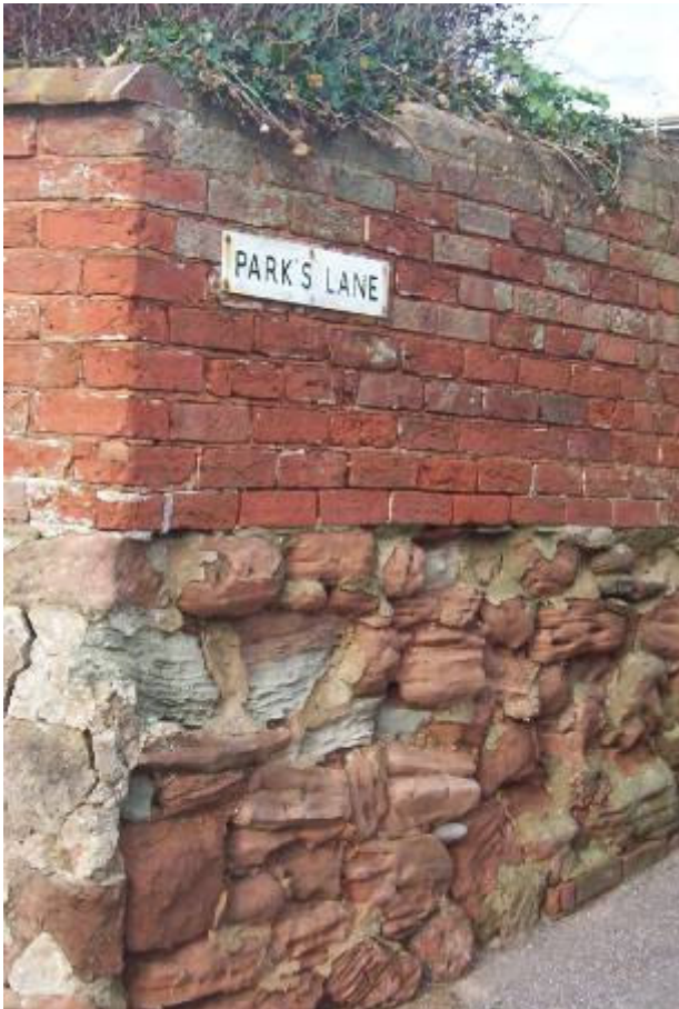
Weathered sandstone and brick wall on the corner of Parks Lane and the cliff path.
