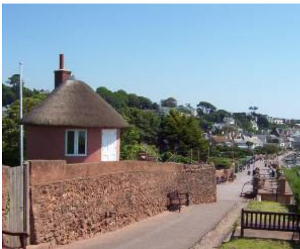
Cliff path with circular gazebo on the garden of a villa. Note the deterioration of the base of the sandstone wall.
