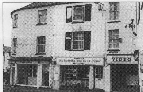
South Street/Lyme Street area show indications of low maintenance, under-use, poor frontage detail, unsightly gaps etc. and are suggestive of a need for grant-assisted enhancement (e.g. a Conservation Area Partnership Scheme)
