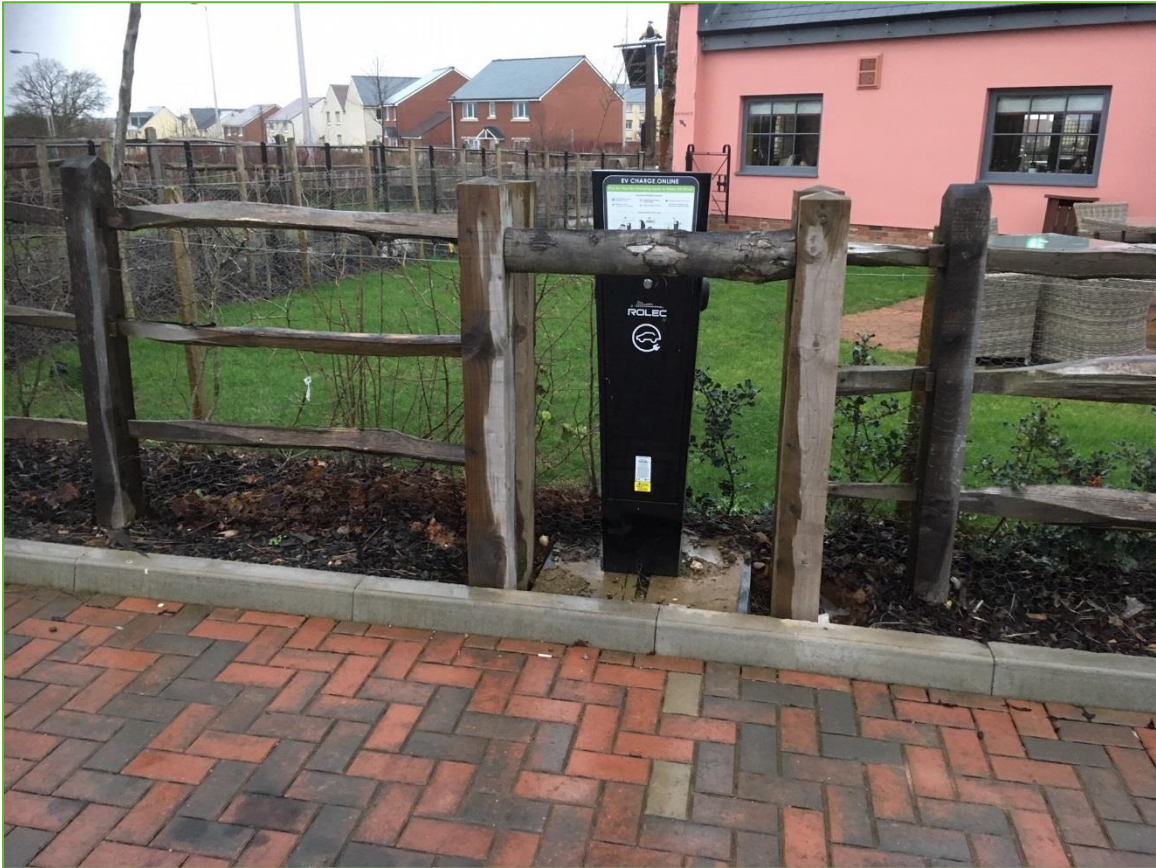
Figure 10 – existing EV charging at Cranberry Farm, Cranbrook
