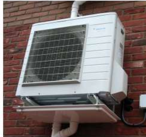
Air source heat pumps are mounted directly on an external wall to make use of the ambient air as a heat source
