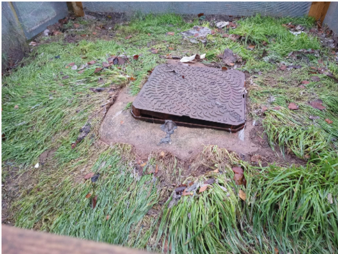
Sewer Flooding Maer Nature Reserve
