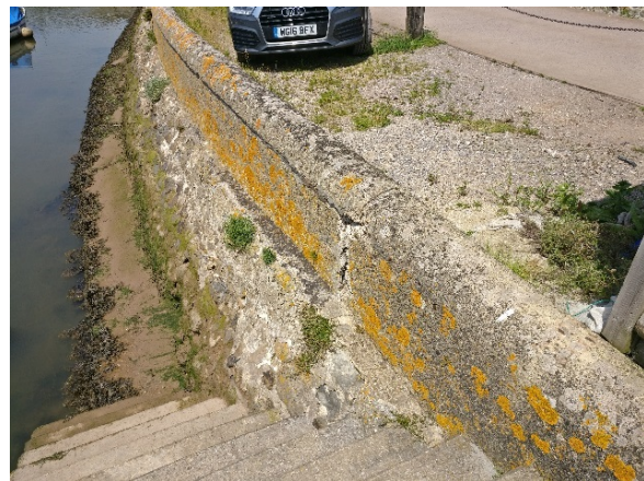
Some vertical cracking of the upper concrete wall
