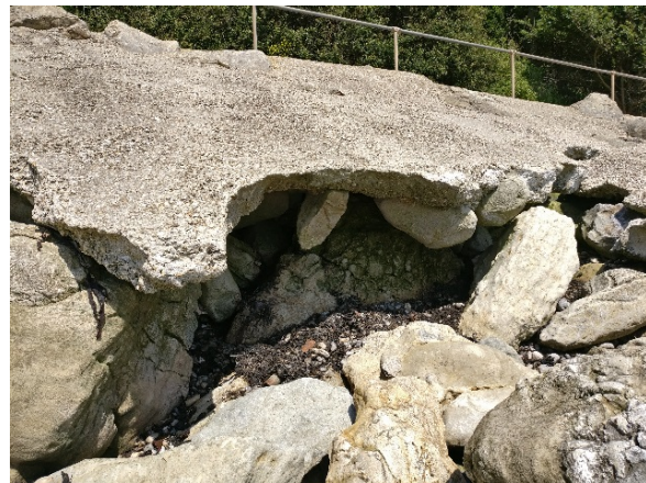
Failure at slope toe leading to loss of fill
