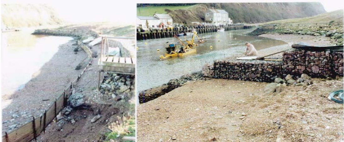
Figure 2-11 Photos of the protective fencing undermined and the construction of the gabion groyne Source: Axmouth Harbour Management (2003)
