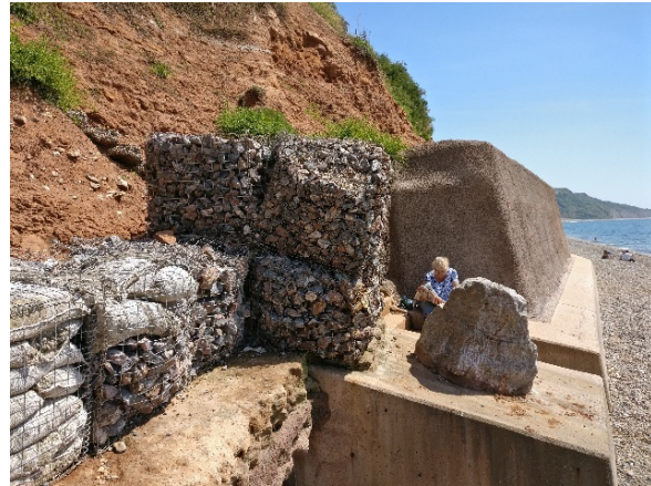
Deformation of gabion baskets and loss of fill material
