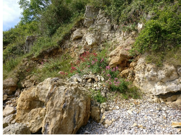
Signs of recent slips with large and small rock
