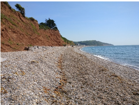
Rock revetment buried in some areas as beach levels increase in elevation
