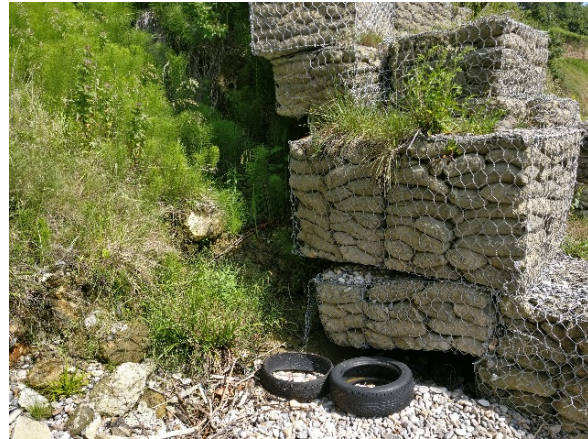
Undermining and outflanking have caused slumping
