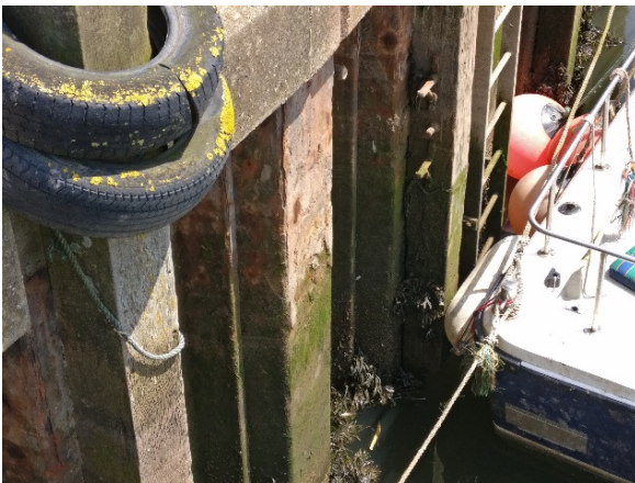
Surface corrosion of the main sheet pile wall
