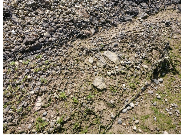
Some damage to steel has allowed loss of fill material
