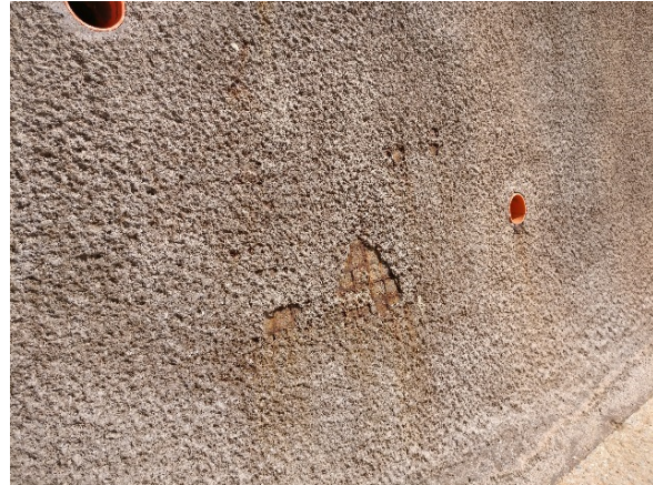
Spalling of surface concrete resulted in exposure of underlying steel
