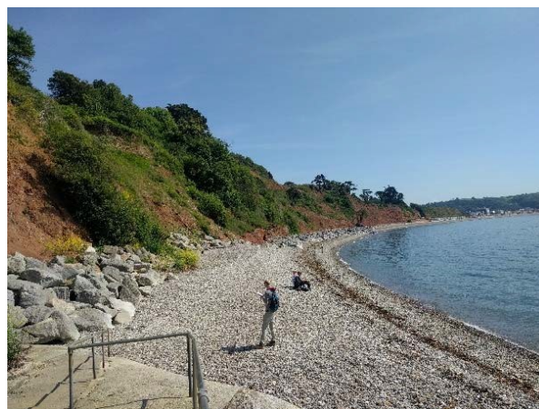
Figure 4.8 Photograph of beach between Seaton Hole and West Seaton Photograph taken during defence condition assessment 28 th June 2017, looking east
