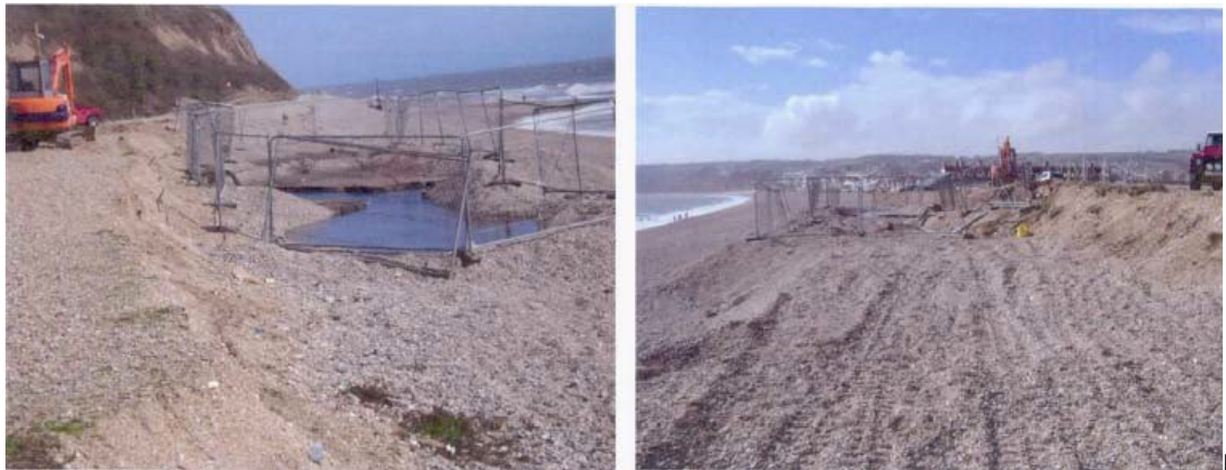
4.22 Trench for disposal of dredge material 2009/2010 Source: Author unknown 0, no date specified
