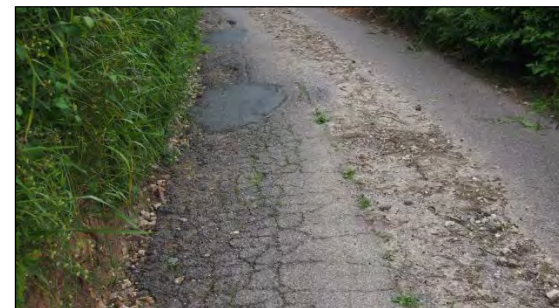
Damaged road surface, Otter Valley
