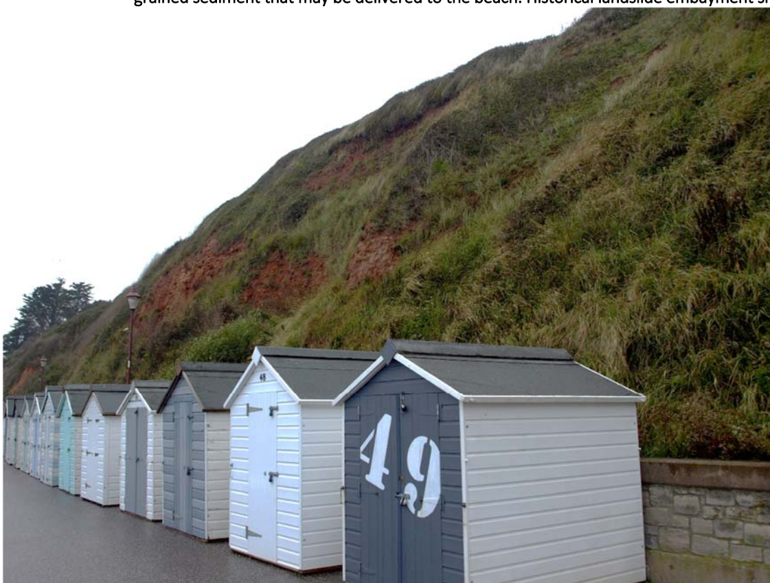
Figure 4i. CBU 7. West Walk. Mudstone cliffs with promenade toe protection since early 1900s. Localised failures on the cliff produce fine grained sediment that is not delivered to the beach.
