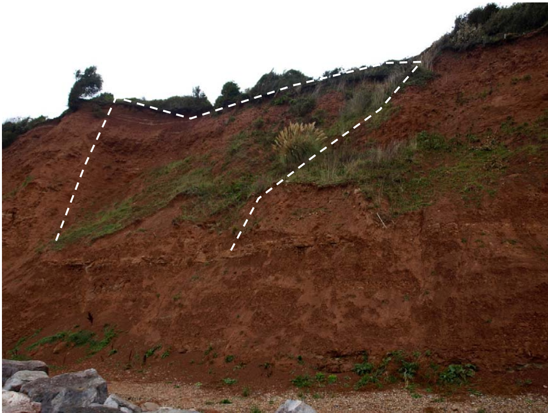
Figure 4f. CBU 4. Seaforth Lodge. Mudstone cliffs with toe revetment largely obscured by beach sediment and debris. Periodic, localised failures produce fine grained sediment that is delivered to the beach. Historical landslide embayment shown.
