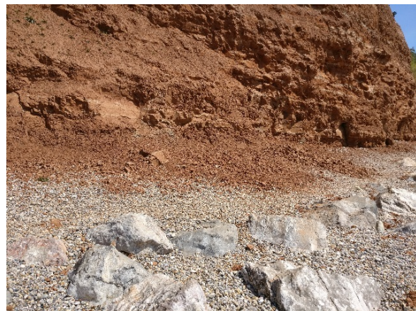
Signs of recent cliff failure behind buried rock revetment
