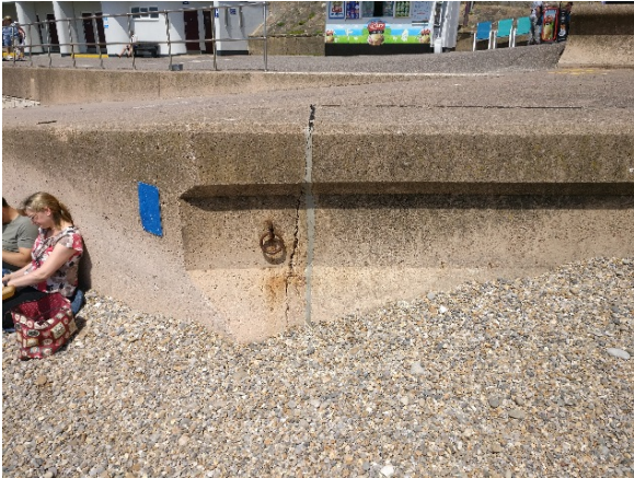
Vertical cracking of concrete seawall with wave return
