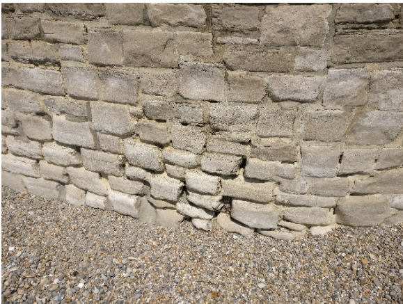
Localised loss of grouting between stone blocks
