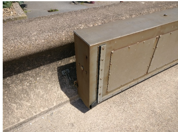
Multiple flood gates present, with damage to rubber seals
