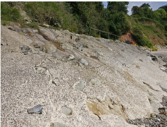
Steep, concrete revetment surface was cracked
