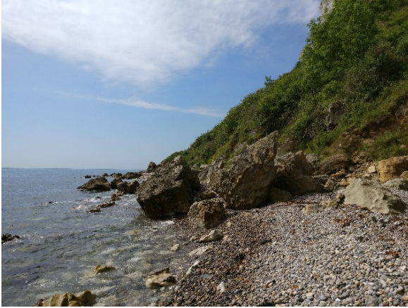
Well-vegetated area of spalled rock at cliff base
