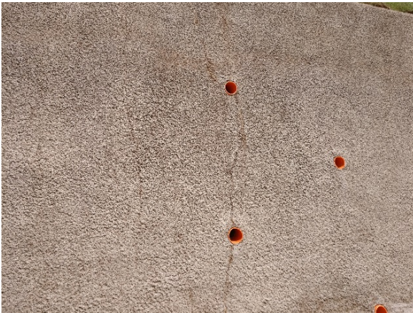
Vertical cracking aligned to drainage channels
