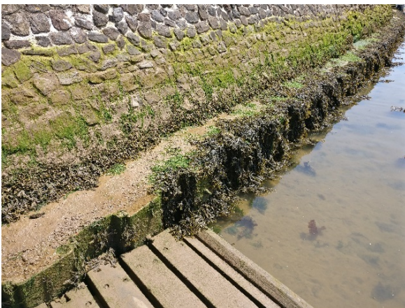
Surface corrosion of steel sheet pile toe
