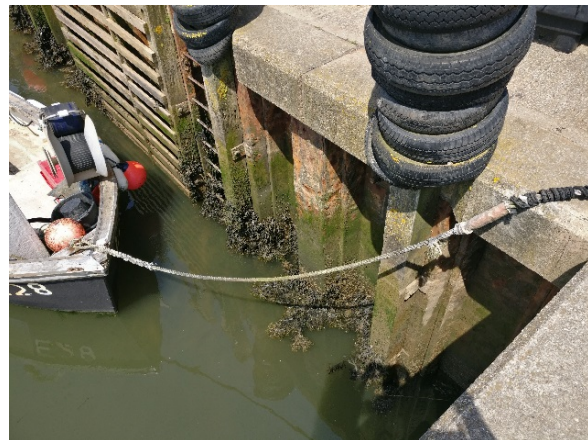
Surface corrosion in the upper section of the sheet pile
