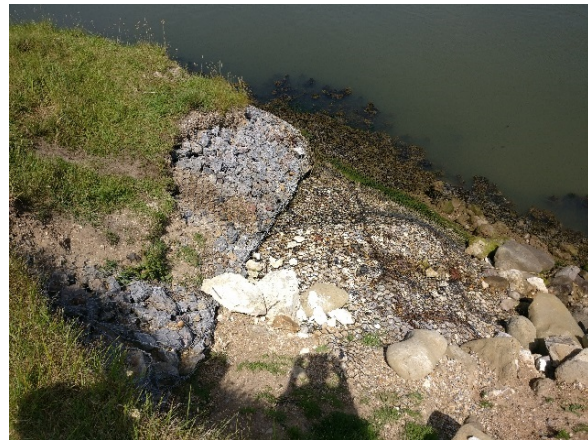
Damage to grass cover and underlying gabion mattresses
