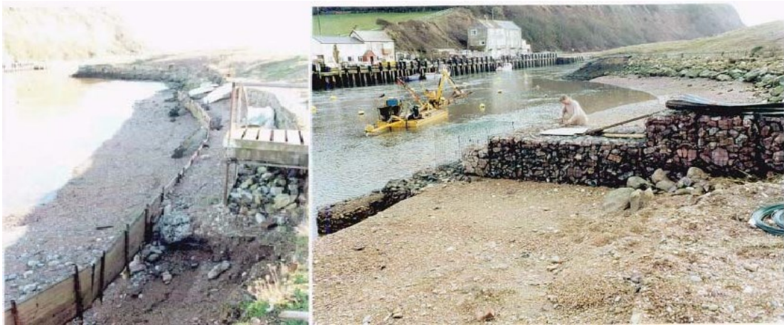
Figure 3-10 Photos of the protective fencing undermined and the construction of the gabion groyne Source: Axmouth Harbour Management Company Ltd, 2003
