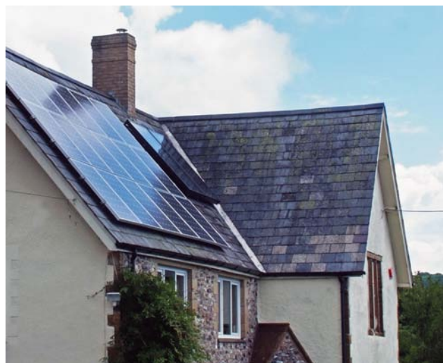
PV and solar panels installed on an older property
