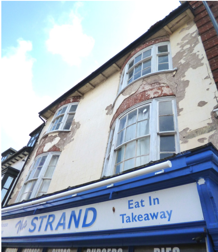
An early nineteenth century grade II listed building with water penetration from blocked gutters.
